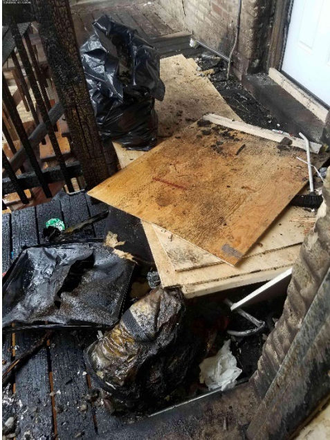
Inspection photograph of rear porch landing with fire damage
