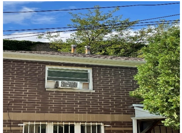
Visible rust on "new" chimney vents.
